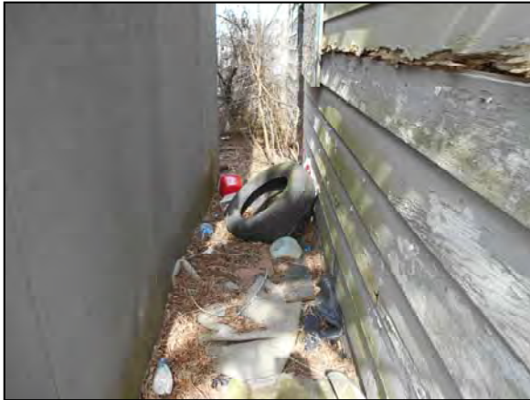
Tire Between Garage and Shed
